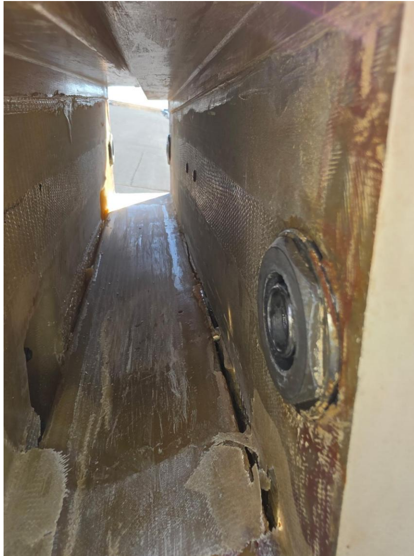
Photograph 2 - View of spar root box crack. (Courtesy of Pilot)
