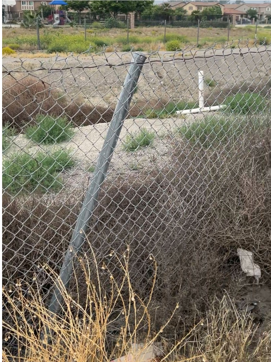
Photograph 5 - Bent fence/post at point of impact (Courtesy of FAA)
