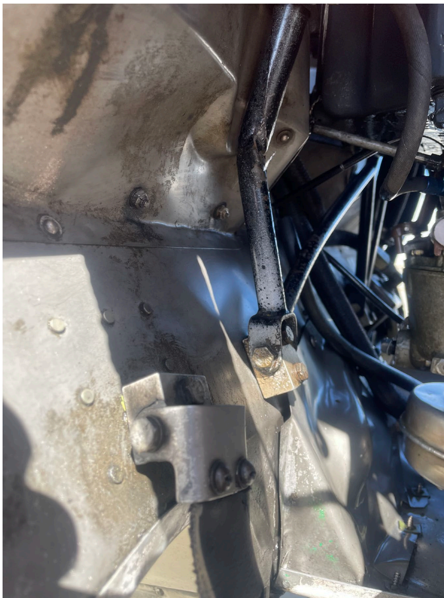
Photograph 2 - View of engine mount damage (Courtesy of Airport Operations)
