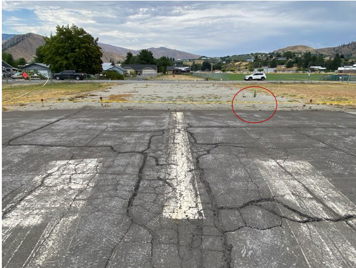
Photograph 3 - Damaged runway end light circled. (Courtesy of FAA)
