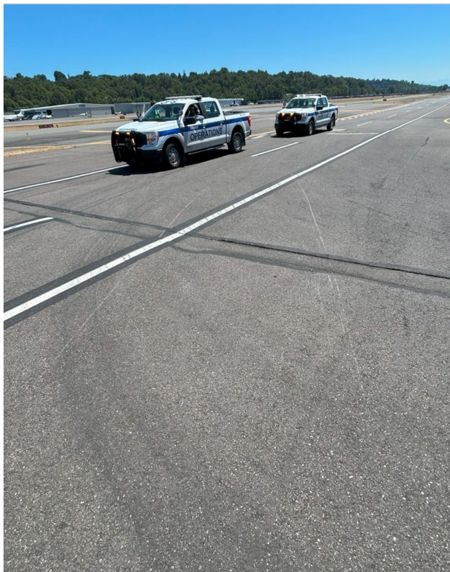
Photograph 3 - Scrapes on ramp surface from helicopter impact. (Courtesy of airport operations).
