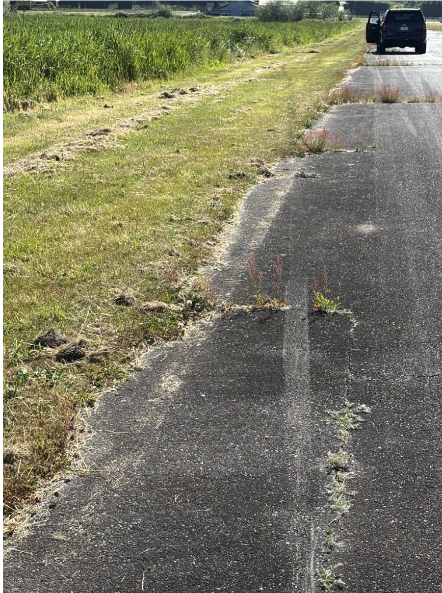
Photograph 3 - View of tire marks along the runway edge. (Courtesy of the FAA.)
