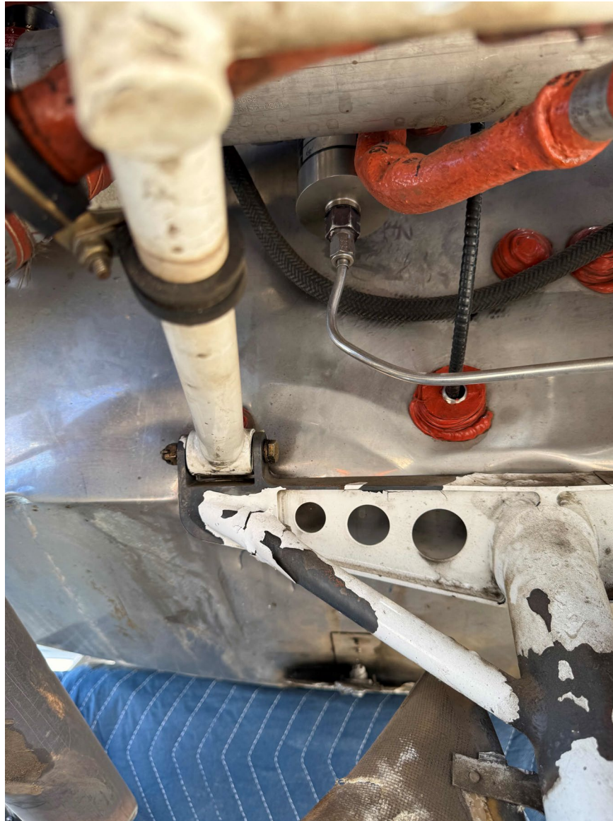
Photograph 3 - View of firewall damage (Courtesy of FAA)
