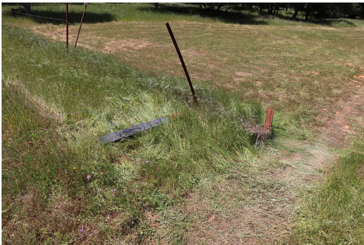
Photograph 3 - View of downed airport perimeter fence post.
