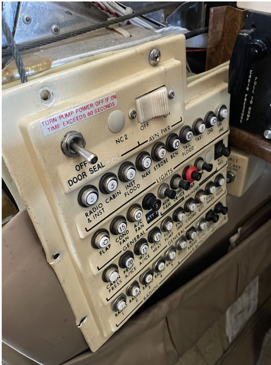
Figure 2. Circuit breaker panel.
