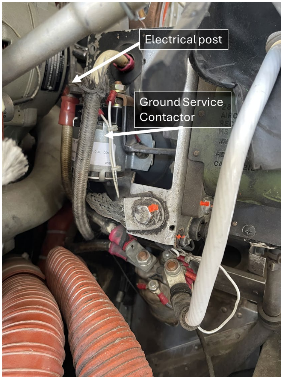
Figure 3. Ground service contactor.
