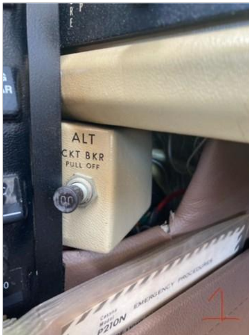
Photograph 1 - Accident airplane, alternator circuit breaker. (Courtesy of the Mechanic)
