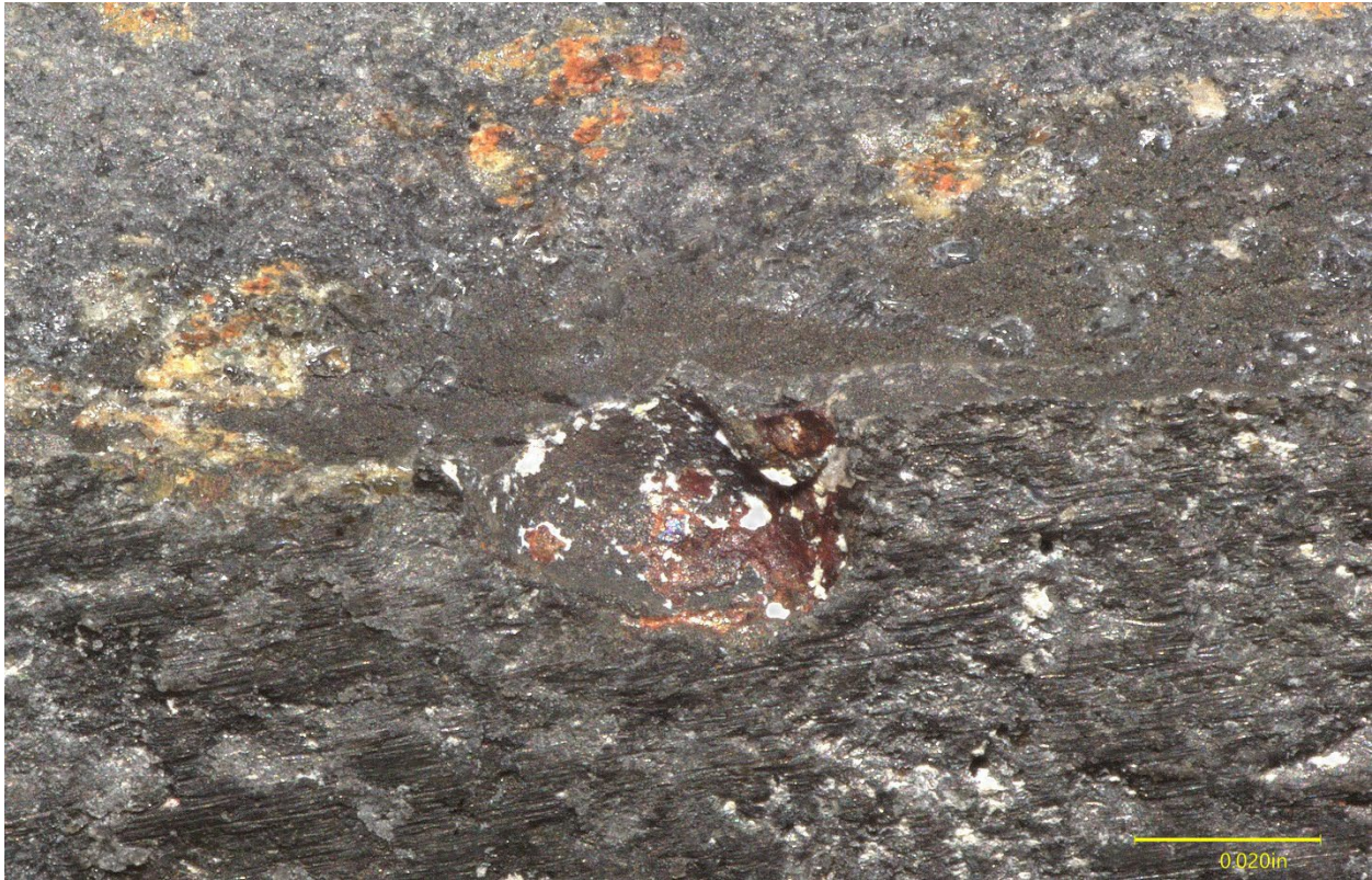
Figure 18. View of the corrosion pit in Figure 17, after chemical stripping of paint.
