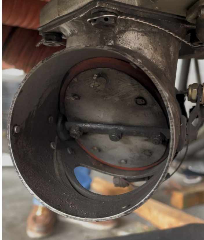
Fig. 4: View of heat door closed in ON position, and cabin control knob at midway limit.
