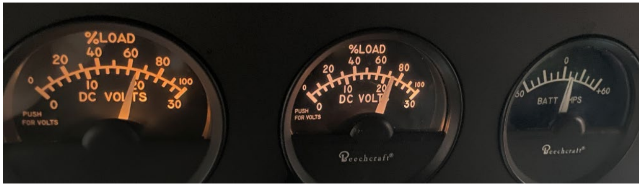
Figure 4: Generator load gauges in overhead panel
