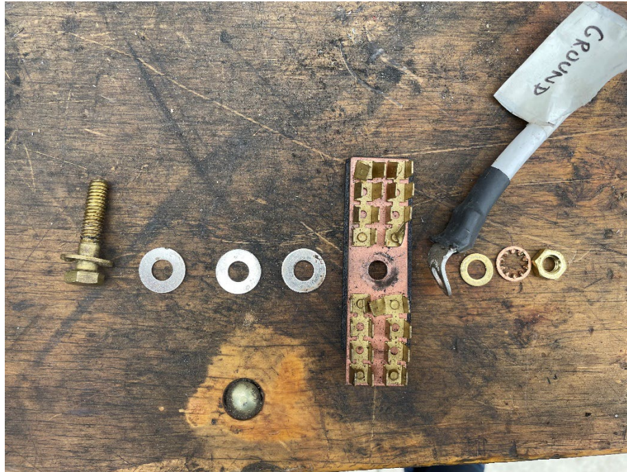
Figure 5. Disassembled feed through stud assembly.
