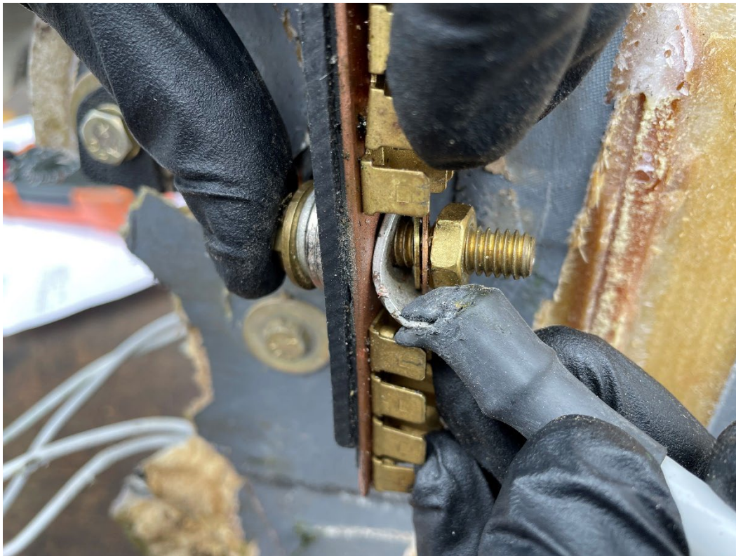
Figure 4. Common ground feed through stud loosely connected to the ground bus.
