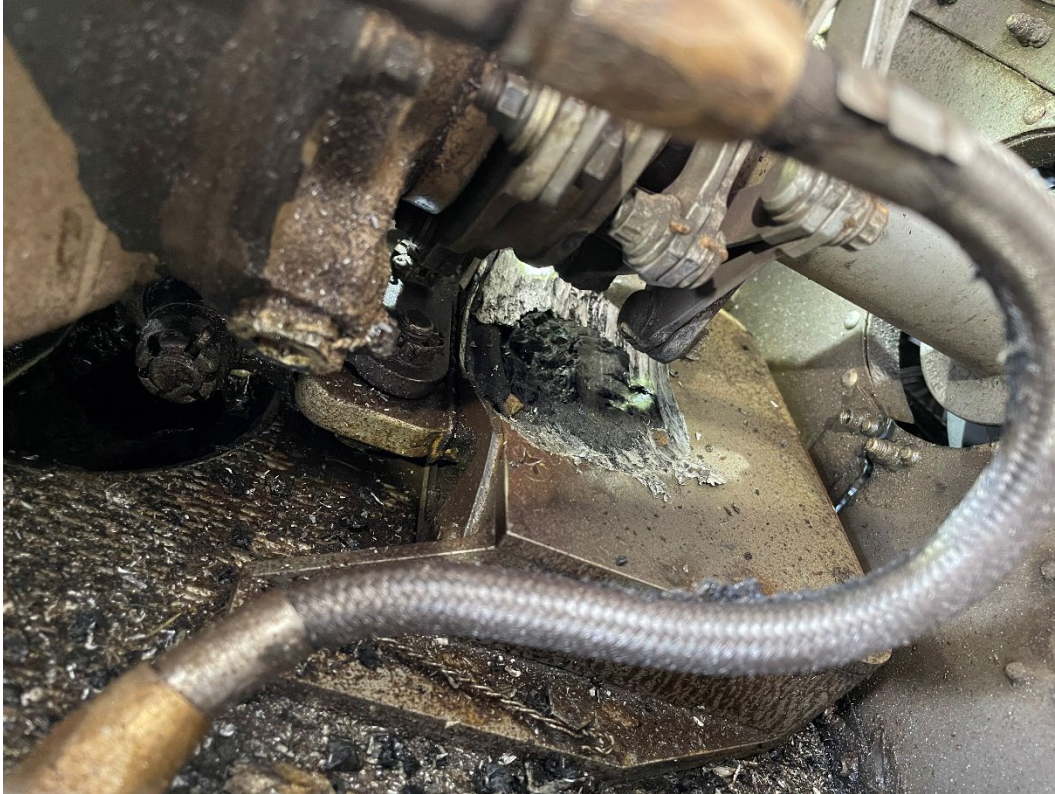
Figure 3. View of isolation mount.
