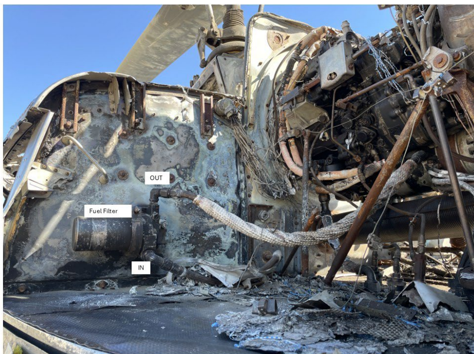
Photograph 2. Engine Side Fuel Filter
