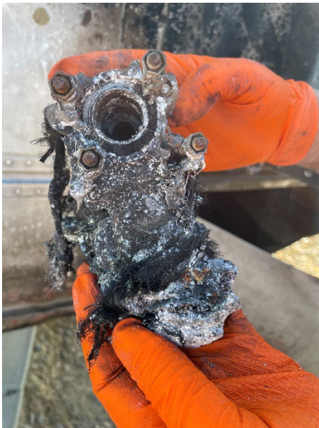
Photograph 6. Top View of Fuel Shutoff Valve
