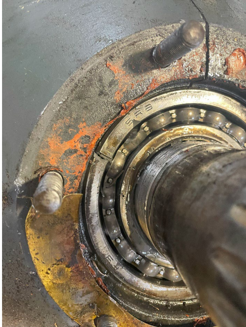
Figure 10. View of roller bearing race.
