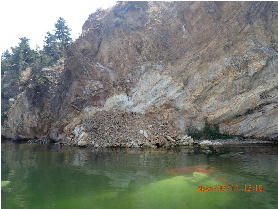
Shoreline Rockface and Debris
