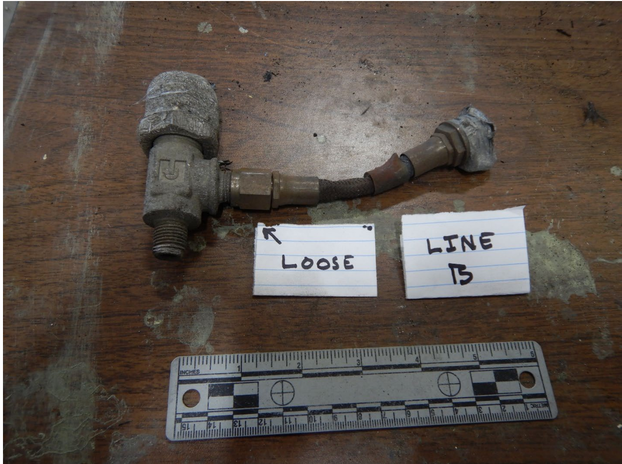
Figure 17. Fuel line B, Pressure relief valve assembly.
