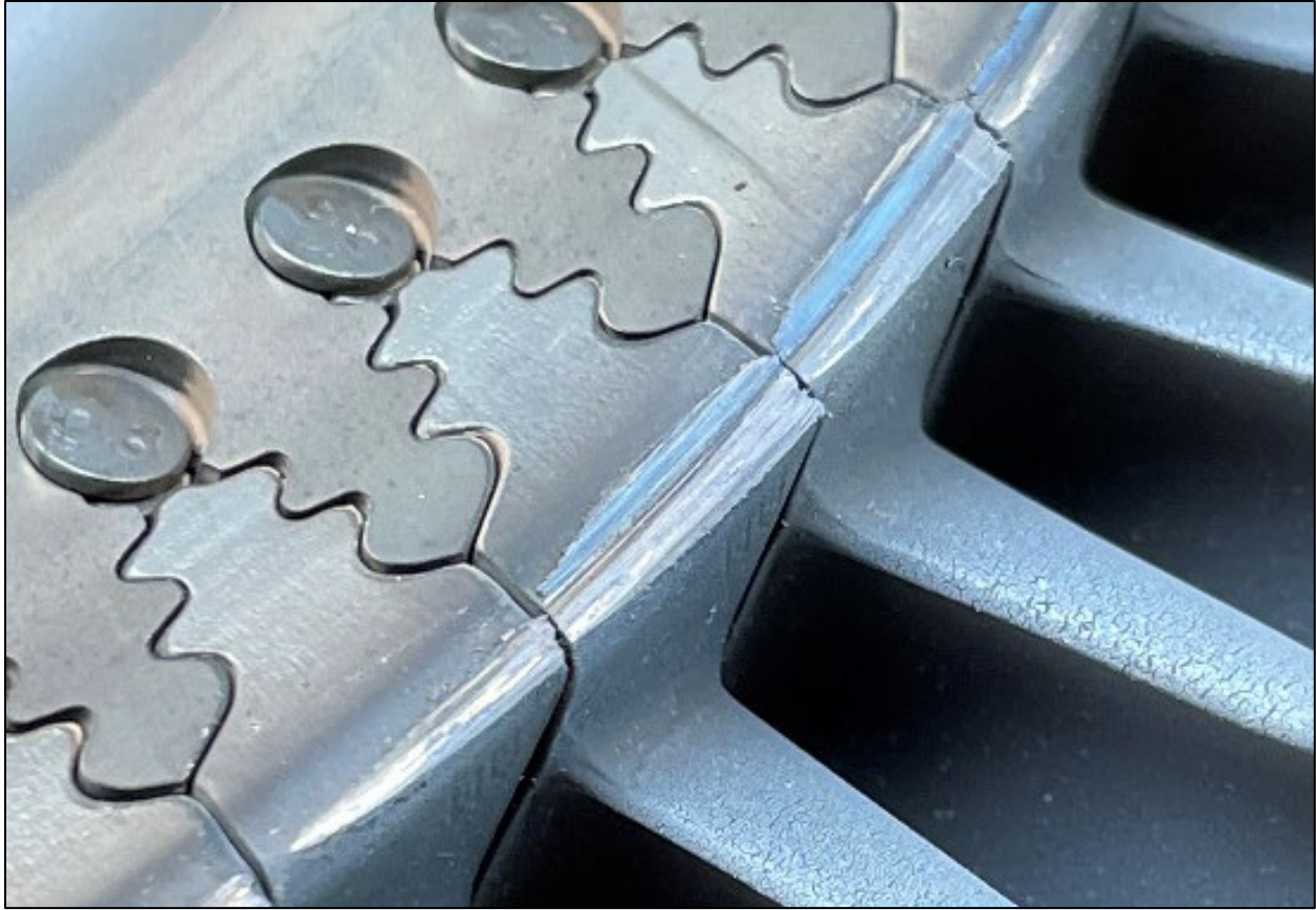
Figure 27. Circumferential rubs on the forward side of CT blade firtrees
