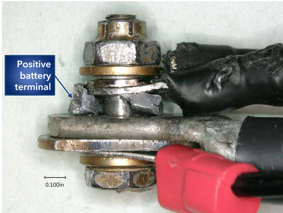
Figure 4. Fracture surfaces on the connection side of the positive battery terminal.
