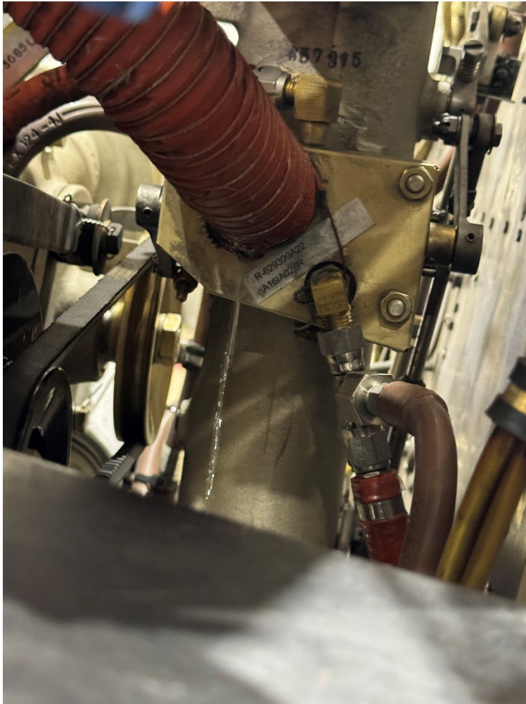
Figure 1: Fuel leaking from the fuel servo outlet line.
