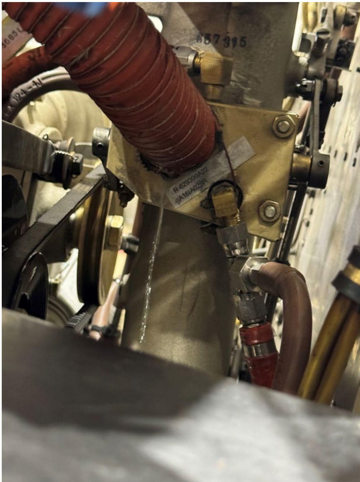
Figure 7. Fuel leaking from the fuel servo outlet line.
