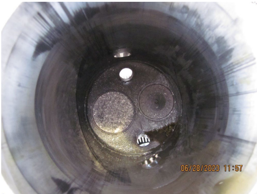
Figure 6: Internal View of No. 1 cylinder barrel
