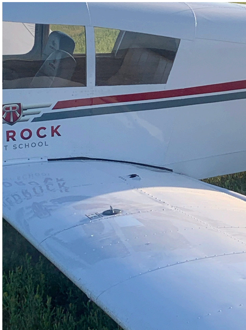
Photo 1 – View of Wing Damage (Courtesy of Pilot)
