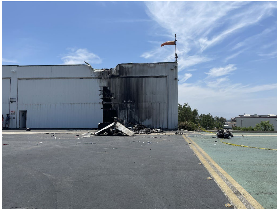
Figure 1. Accident Site Overview
