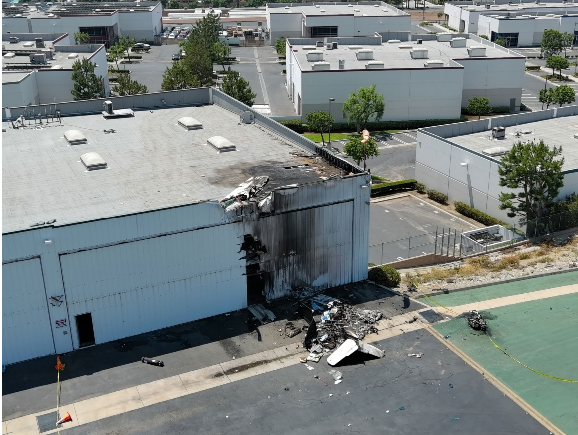
Photograph 1 - Aerial View of Accident Site (Courtesy of Law Enforcement)
