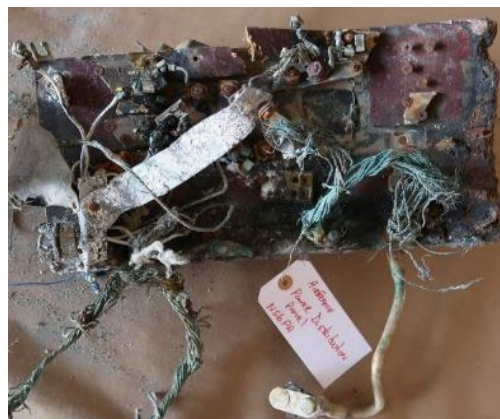
Figure 27. Recovered generator control panel.
