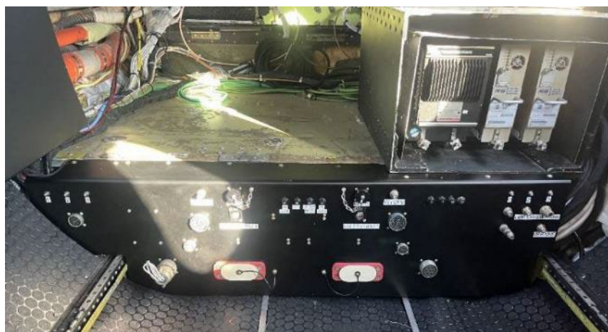
Figure 28. Exemplar photo of the mission equipment J-box located in the very aft area of the airplane cabin. (Source: Phoenix Air Group)
