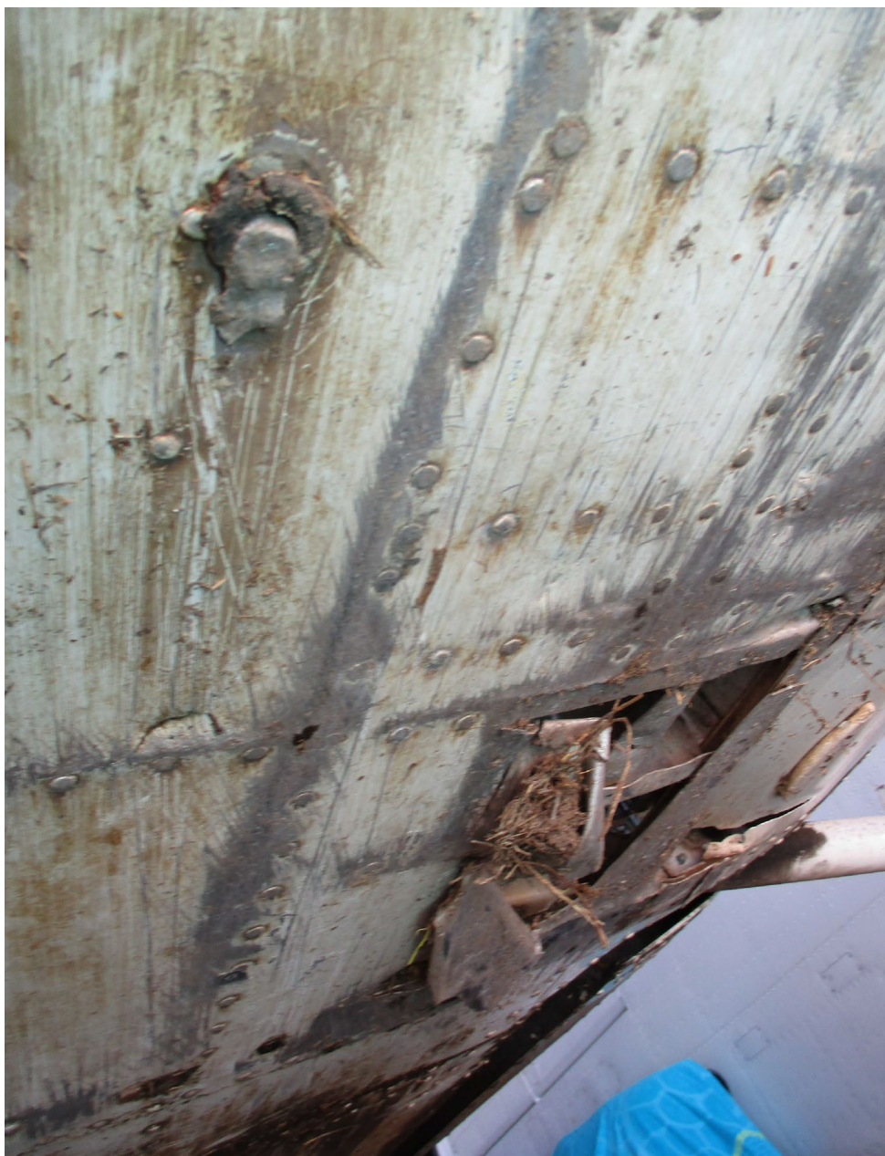
Photo 2 – View of substantial damage (photo provided by pilot)
