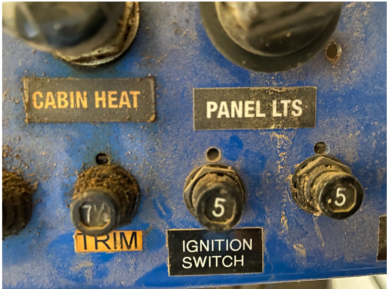
Figure 4. Ignition switch circuit breaker. (Photo courtesy of the FAA)
