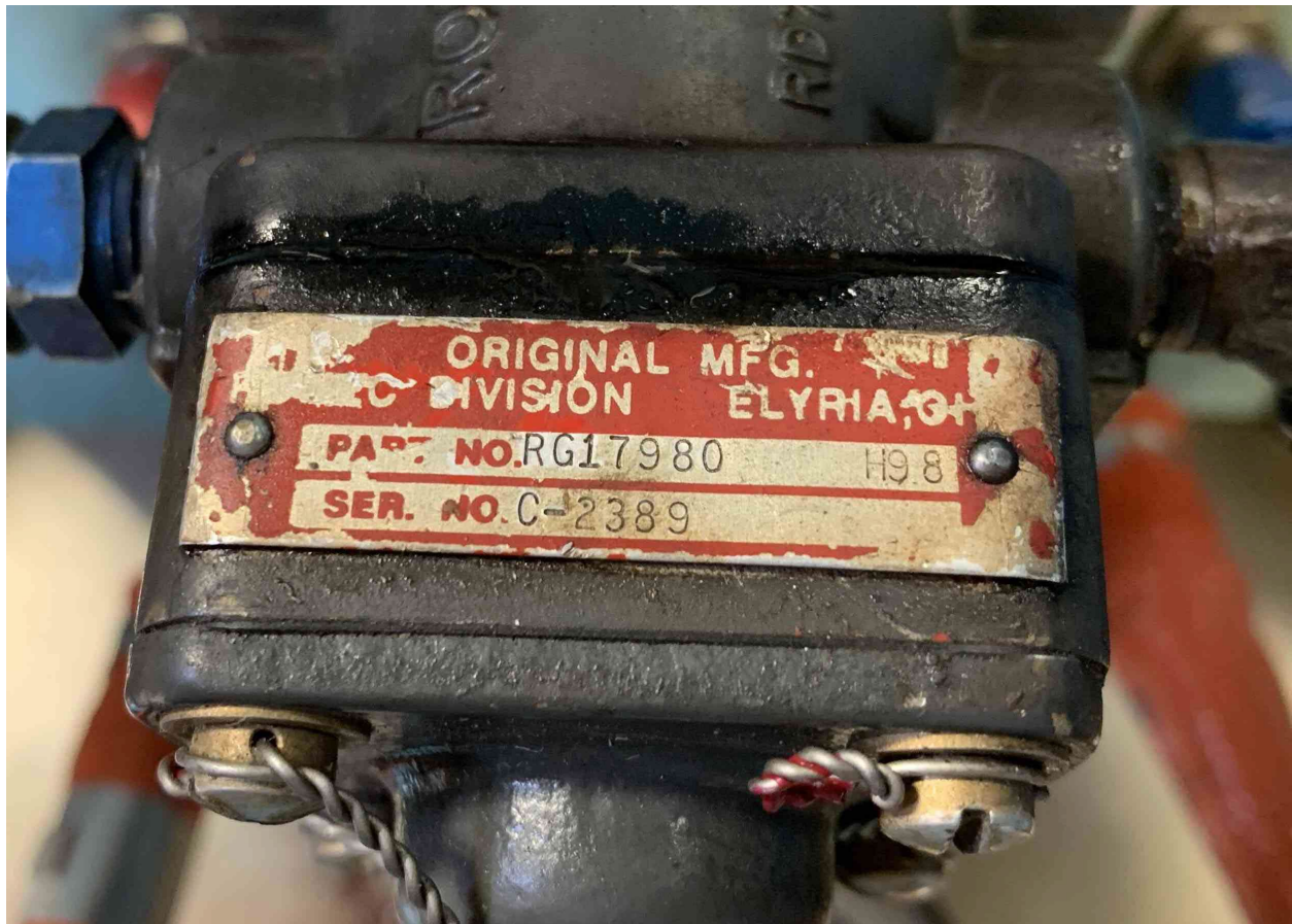
Figure 6 - Fuel leak from split case seal
