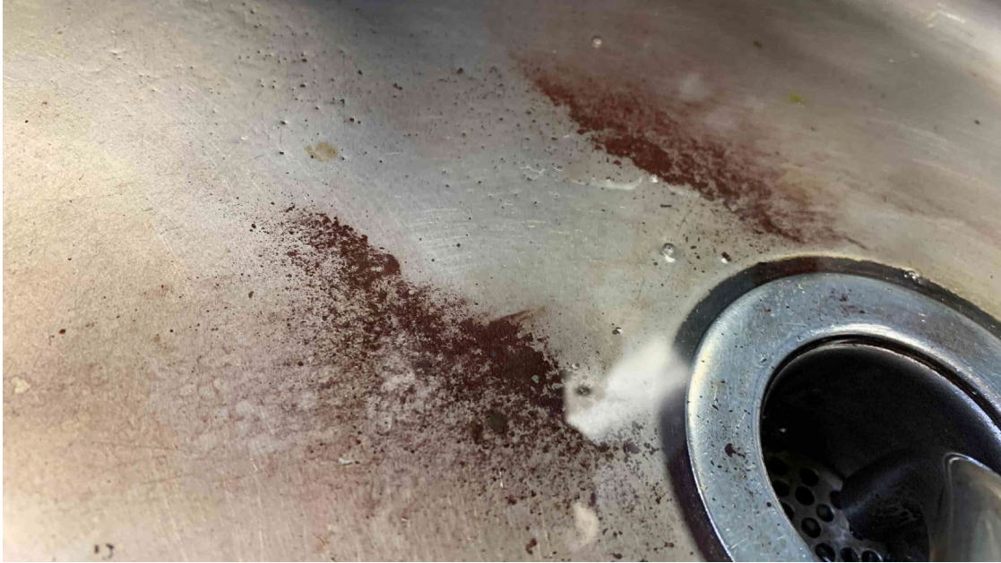
Figure 8 - Corrosion-like deposit from seal drain
