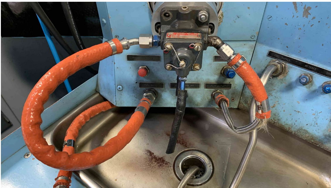
Figure 9 - Kinked output line installed
