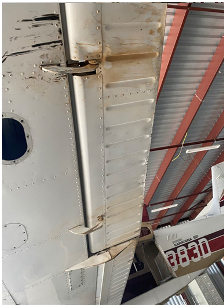
Photo 2 – Underside of the left wing. Photo courtesy of the pilot.
