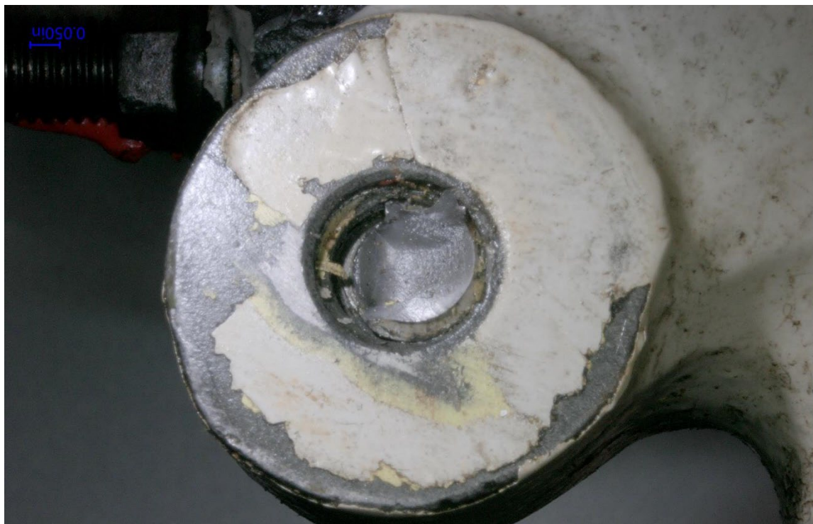
Figure 18. Closer view of the fractured bolt and surrounding housing.
