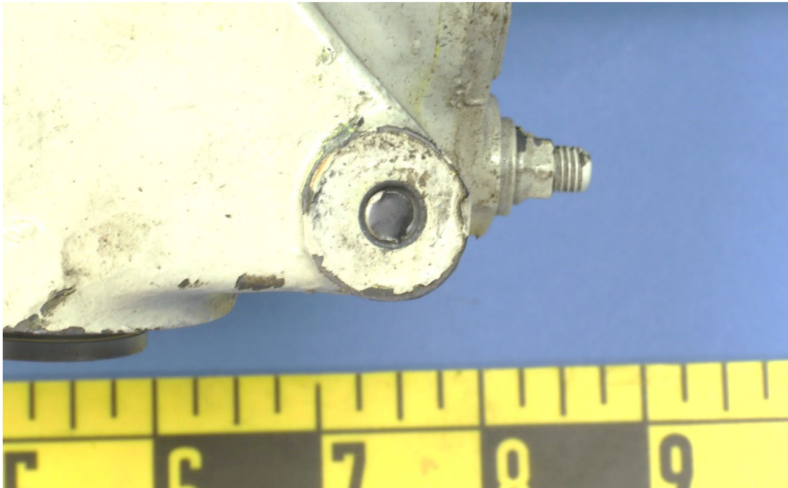
Figure 14. View of the fractured bolt from the aft left (lower right in Figure 7 ).
