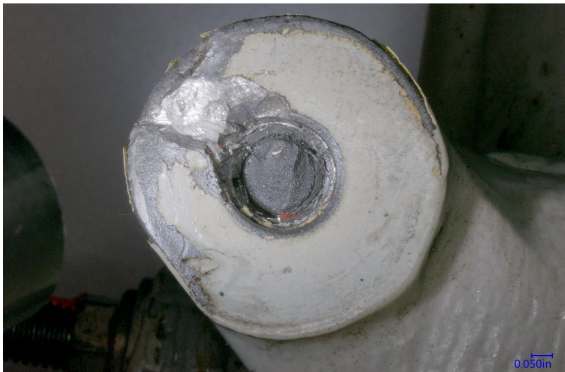
Figure 9. Closer view of the fractured bolt and surrounding housing.
