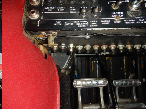
Figure 2 - Popped LG Motor Circuit Breaker
