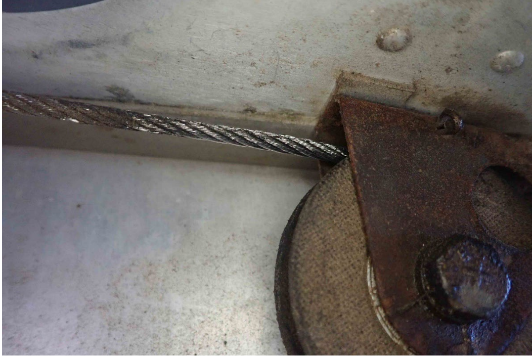
Figure 4 - Right aft rudder pulley and cable
