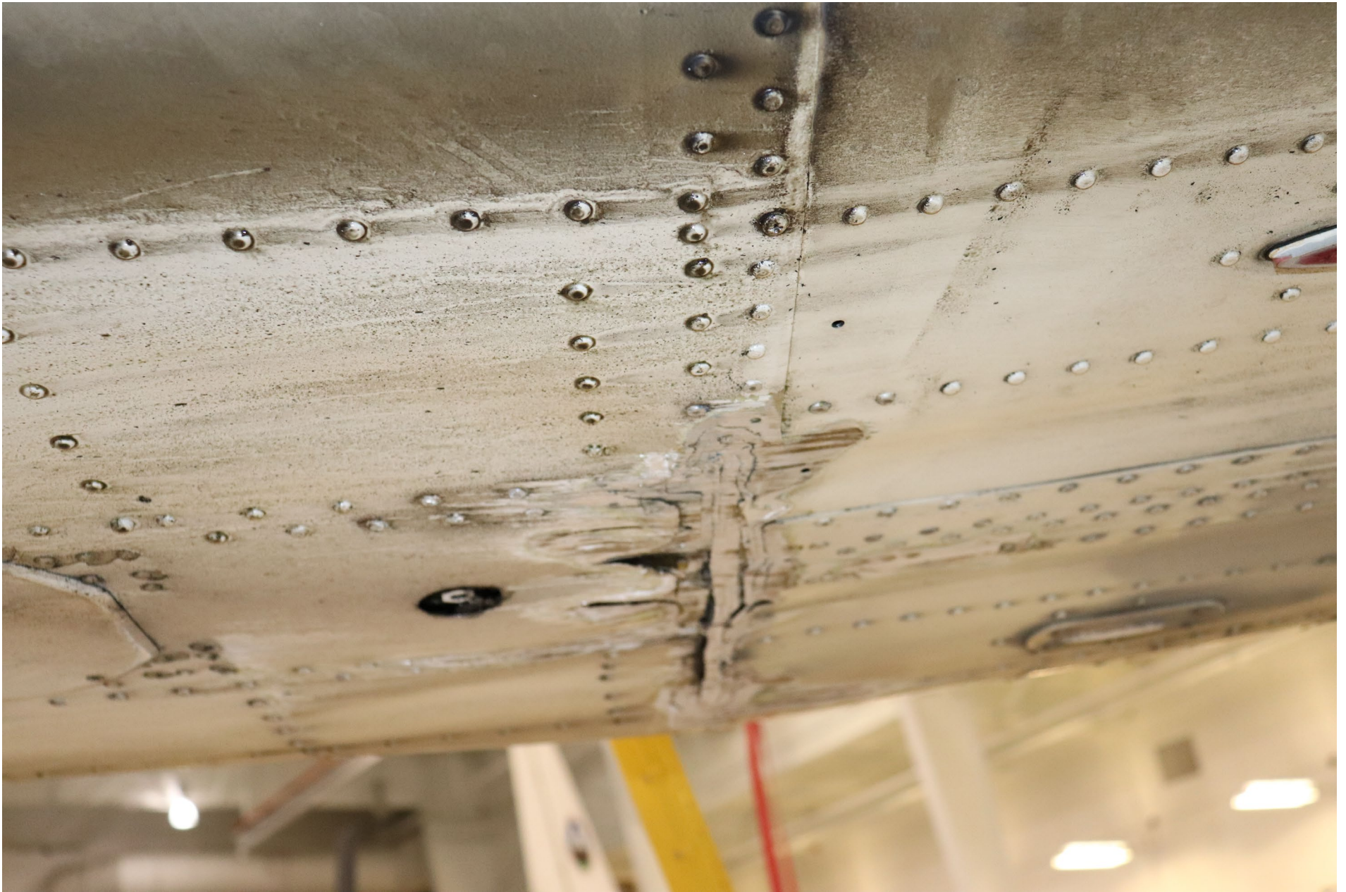
Photo 5 - View of airplane undercarriage damage (photo courtesy of the NTSB)
