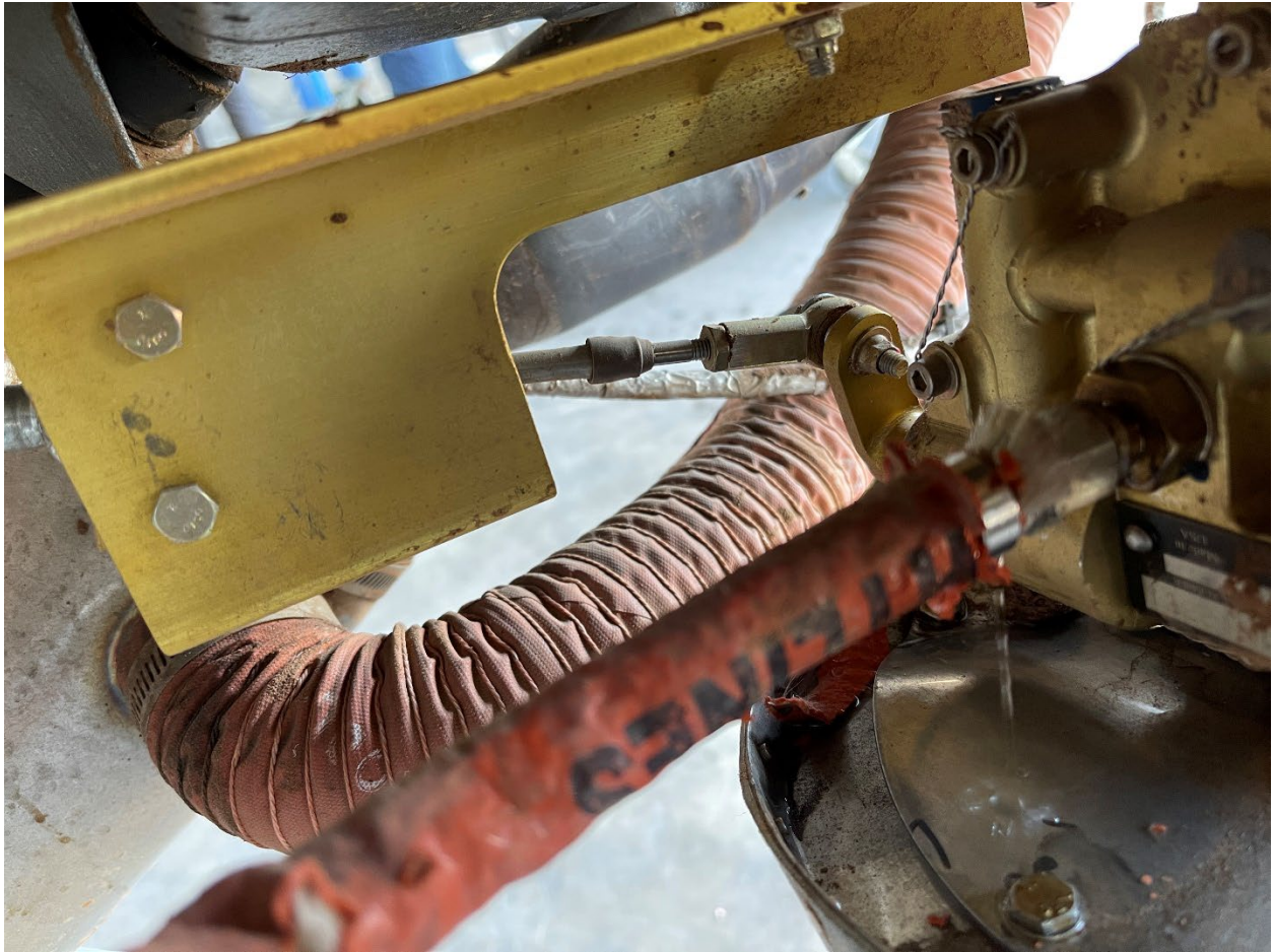
Figure 1: View of the fuel servo outlet fuel line, with fuel leaking.
