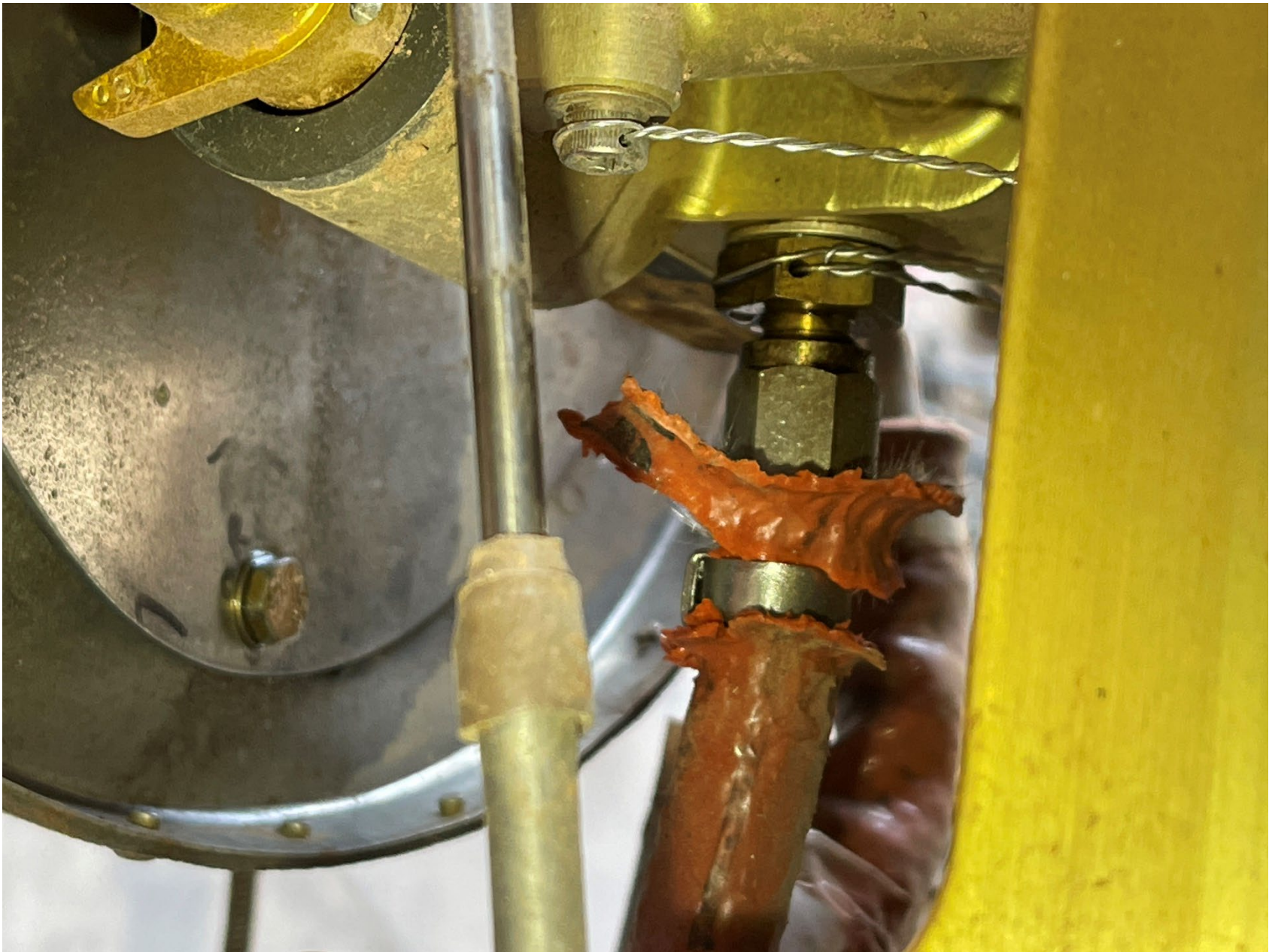
Photo 3 – View of the outlet fuel line at the fuel servo.
