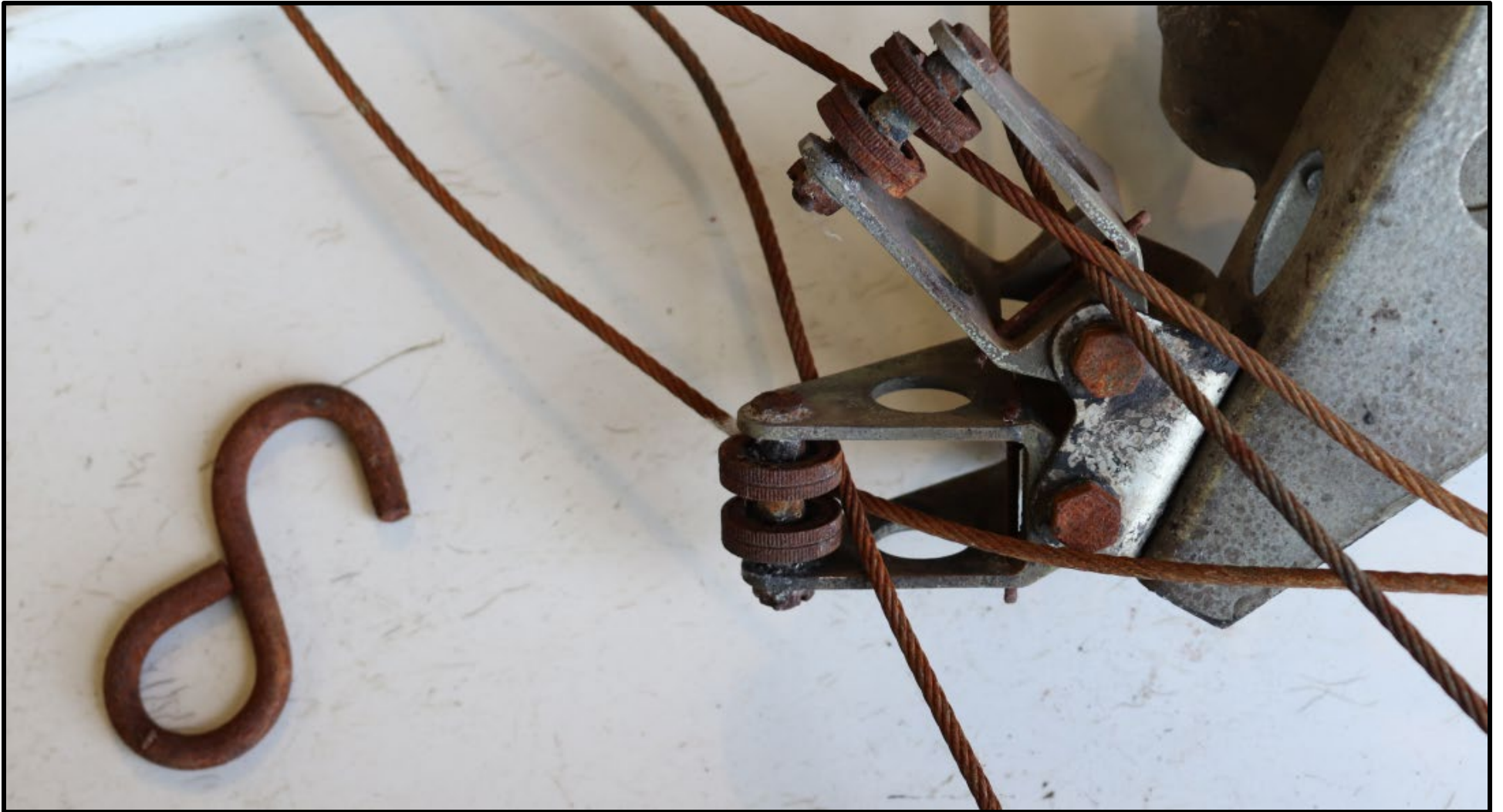
Figure 11: Up-close of No. 9 Pulley
