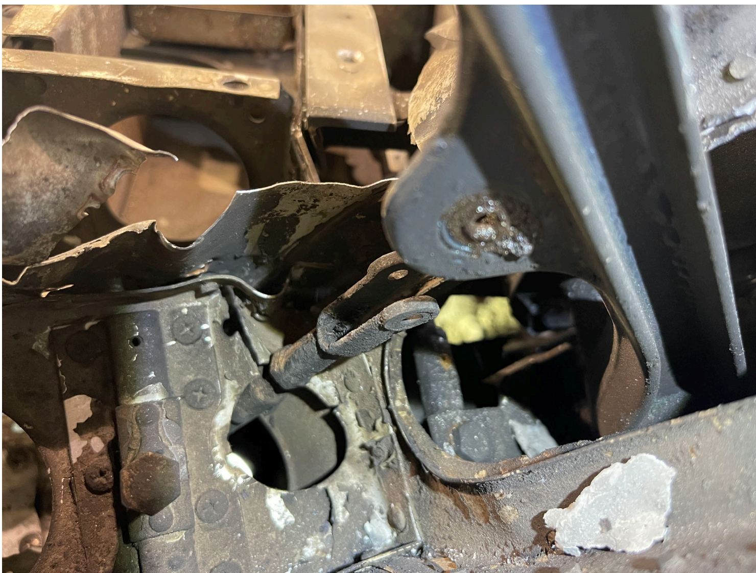
Photograph 7 - Elevator Control Linkages
