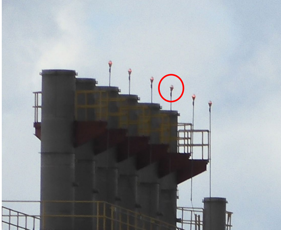
Figure 6. The group of six vent stacks with their aircraft warning lights. Five of the six lights were noted to be illuminated postaccident. The non-illuminated light is circled.
