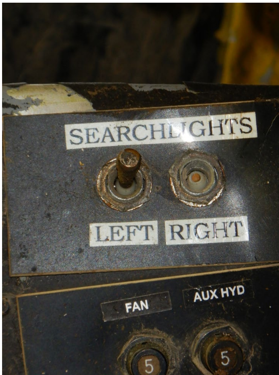
Figure 35. Search lights switches in the ON position.
