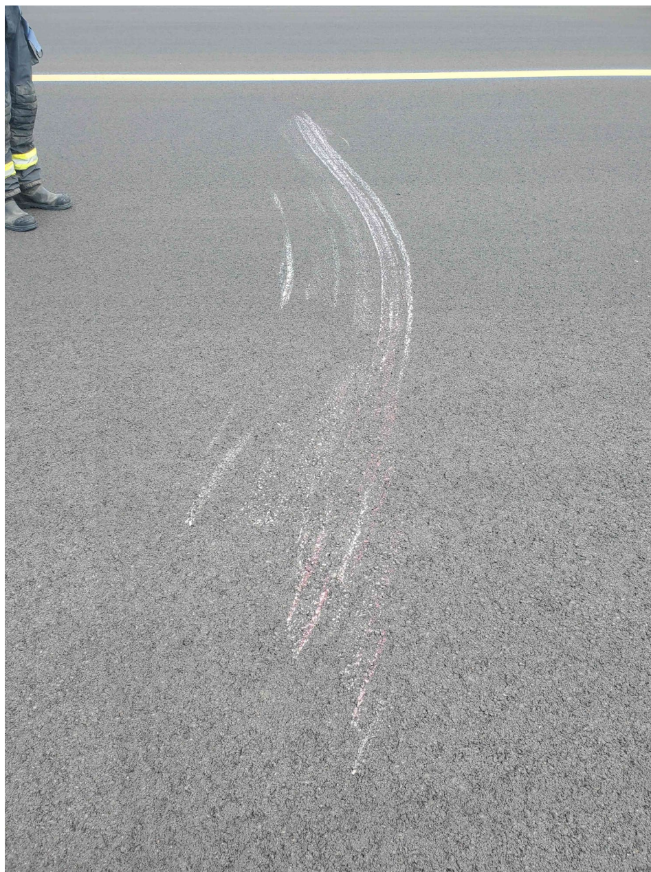
Photo 5 – Wing transfer marks at east runway safety area, taxiway A3
