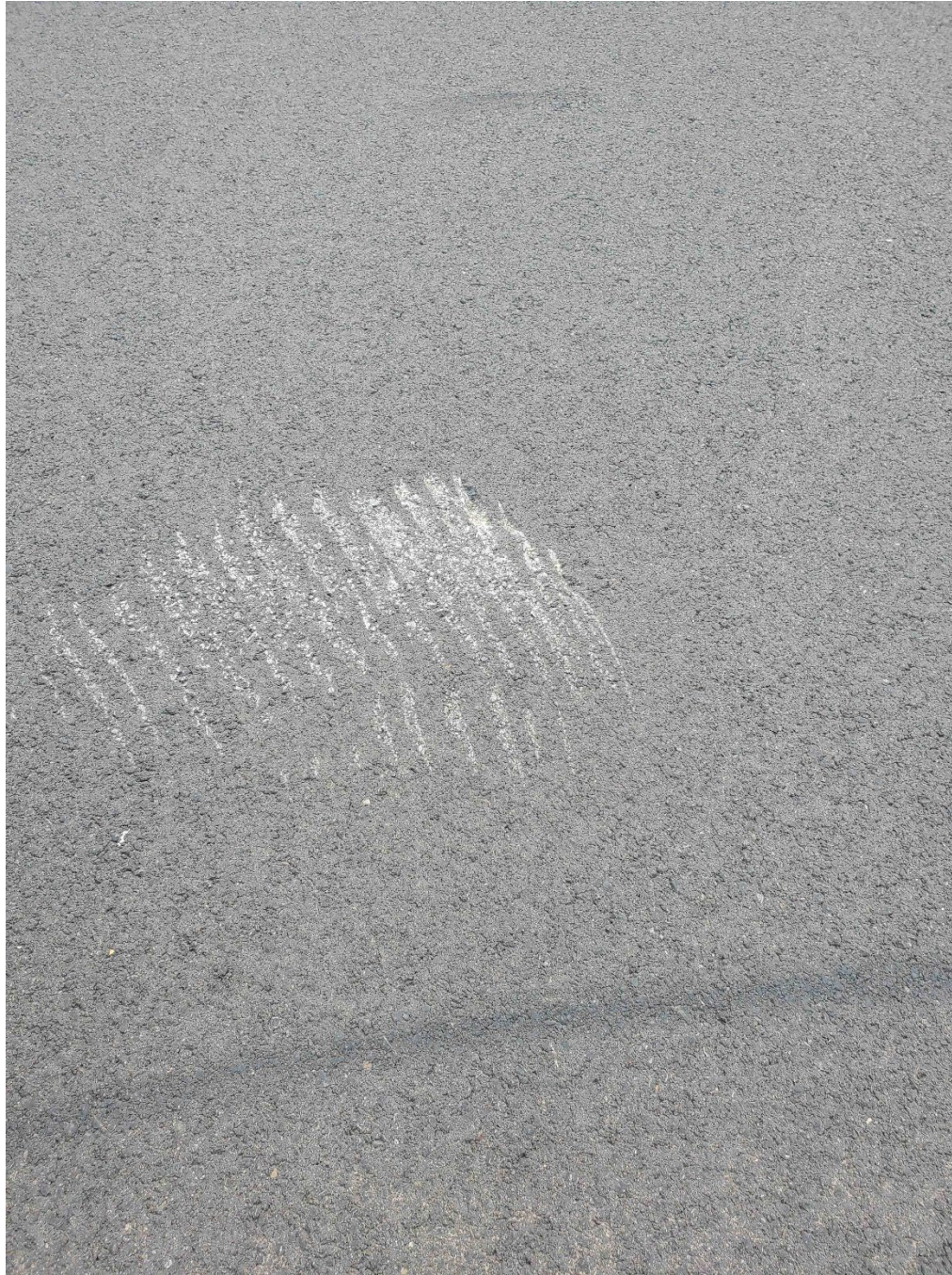
Figure 6 – Propeller blade transfer marks at east runway safety area, taxiway A3
