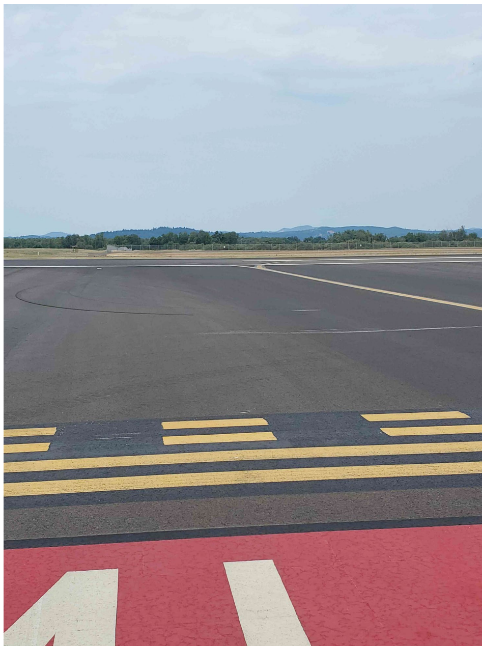
Photo 3 – Tire, propeller, and wing transfer marks at east runway safety area, taxiway A3
