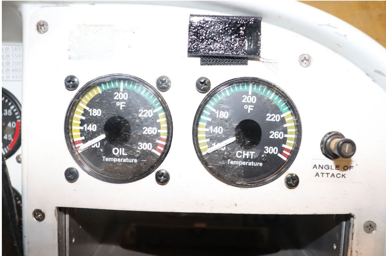
Figure 1. View of cylinder head temperature gauge
