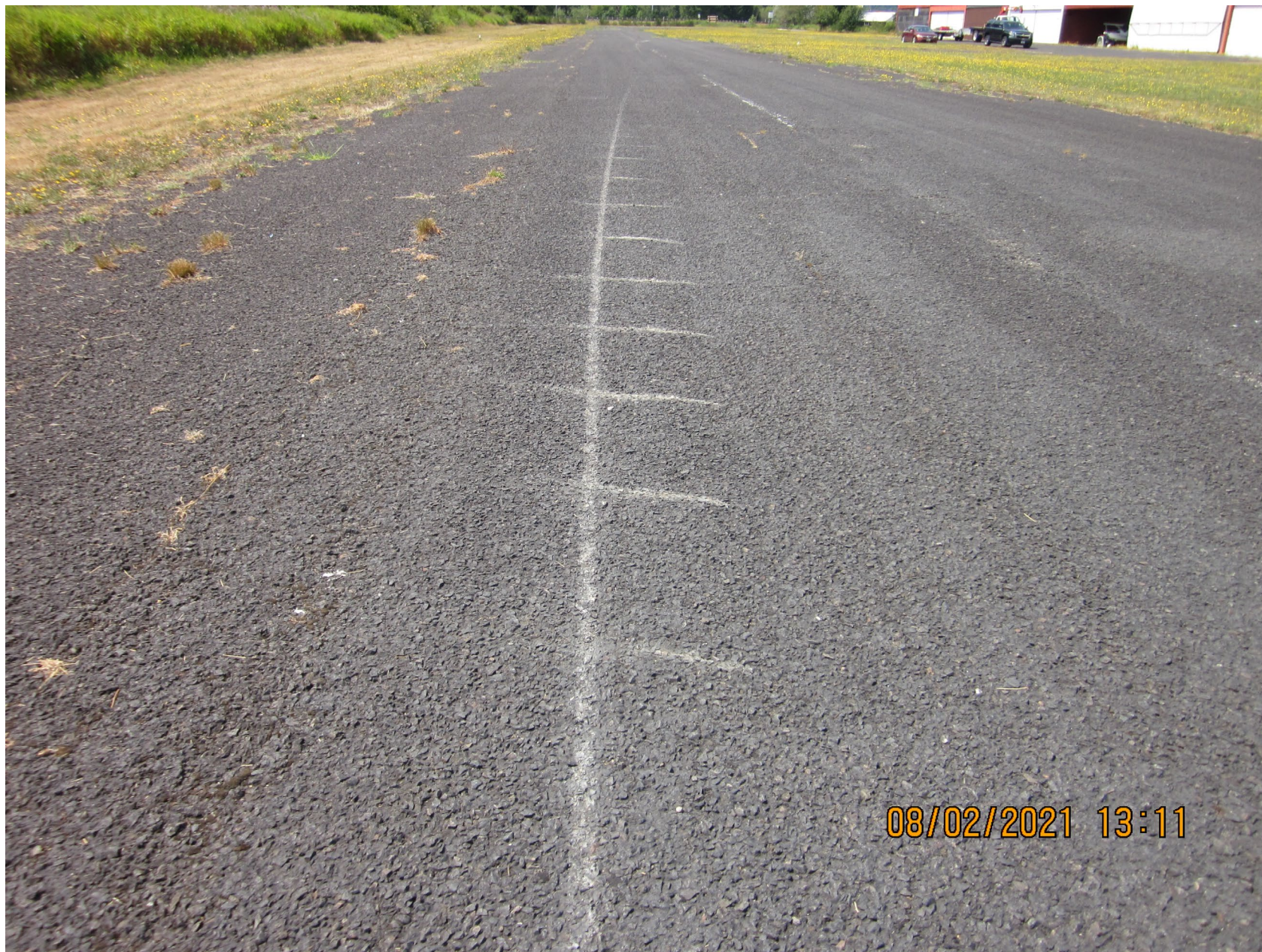
Photo 5 – Prop markings on the runway
