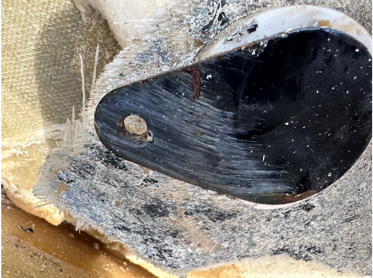
Figure 4. welded plate bent at the tab area with scratch marks
