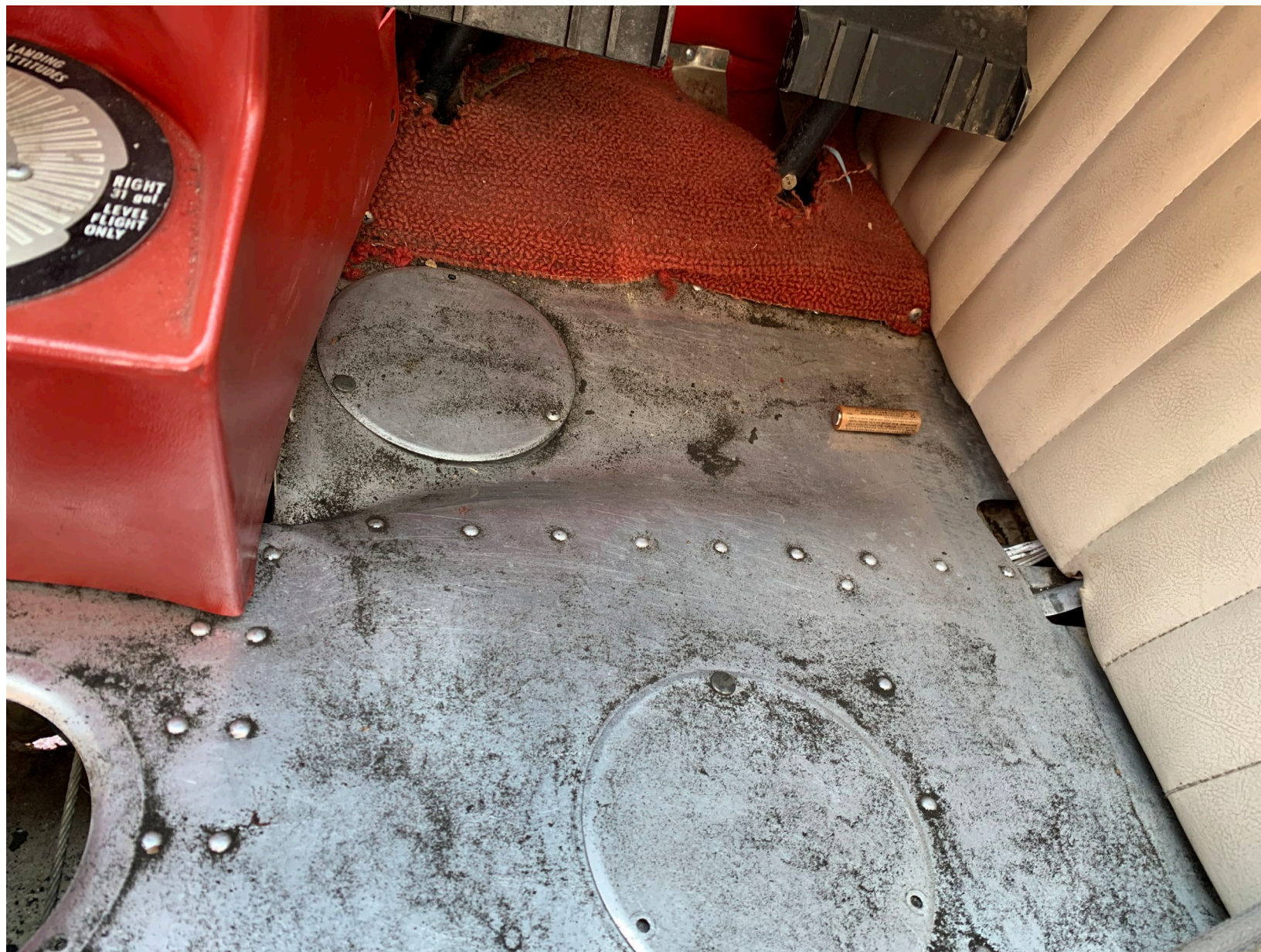
Photo 3 – Buckling at right seat passenger seat floor (Courtesy of Federal Aviation Administration)
