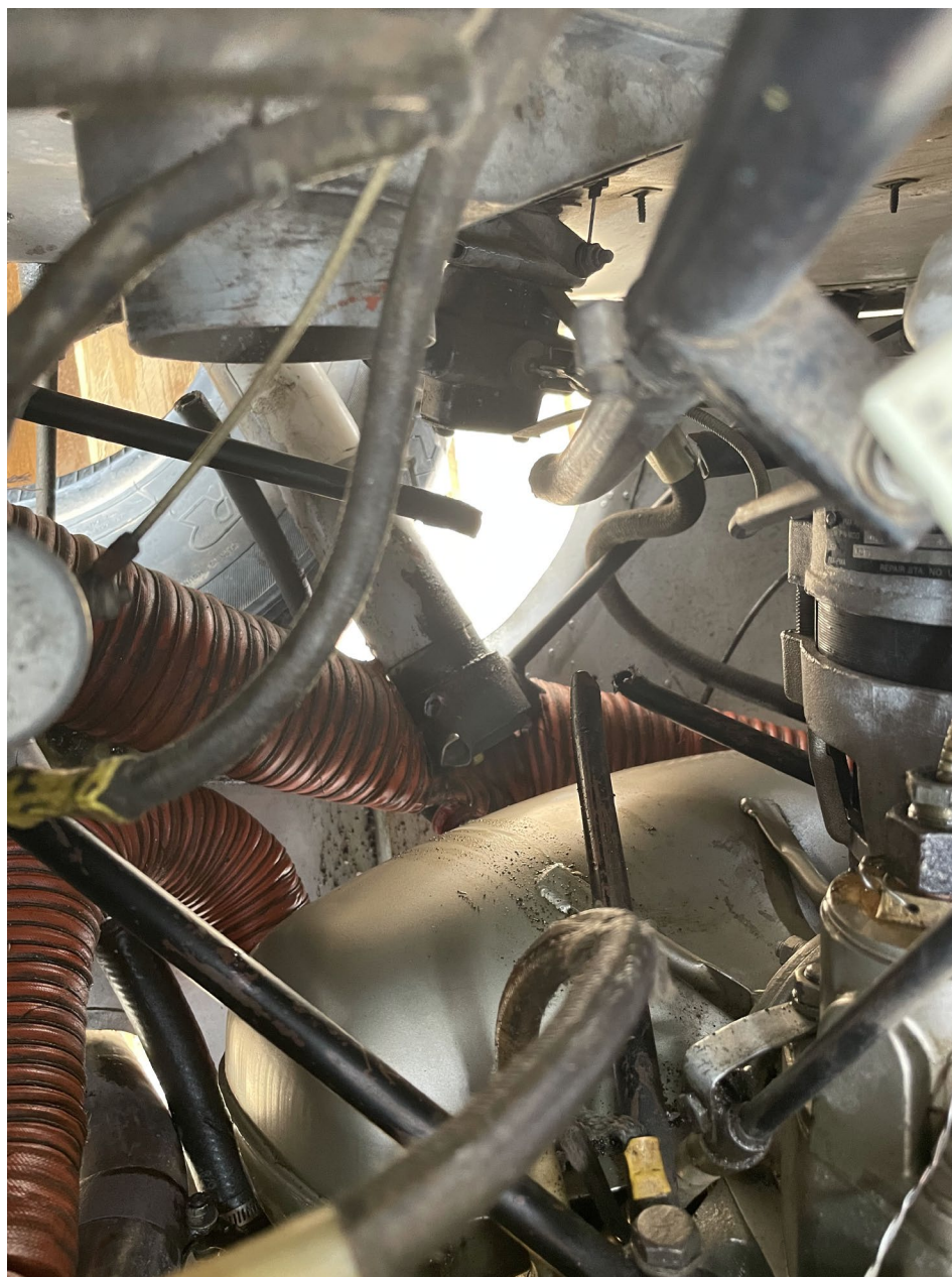
Photo 2 – View of damaged engine truss (courtesy of the FAA)
