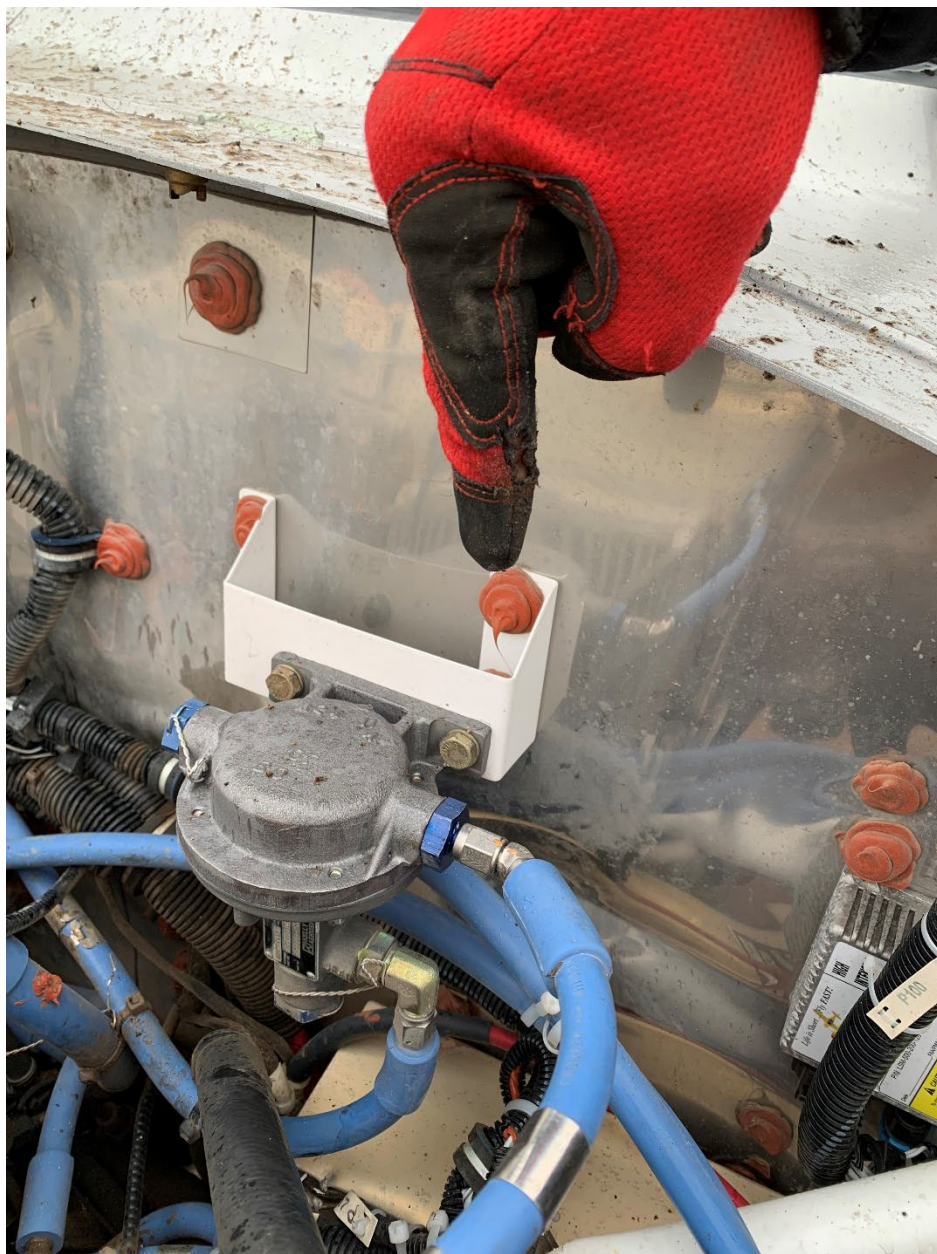
Figure 9. Airline found loose.
