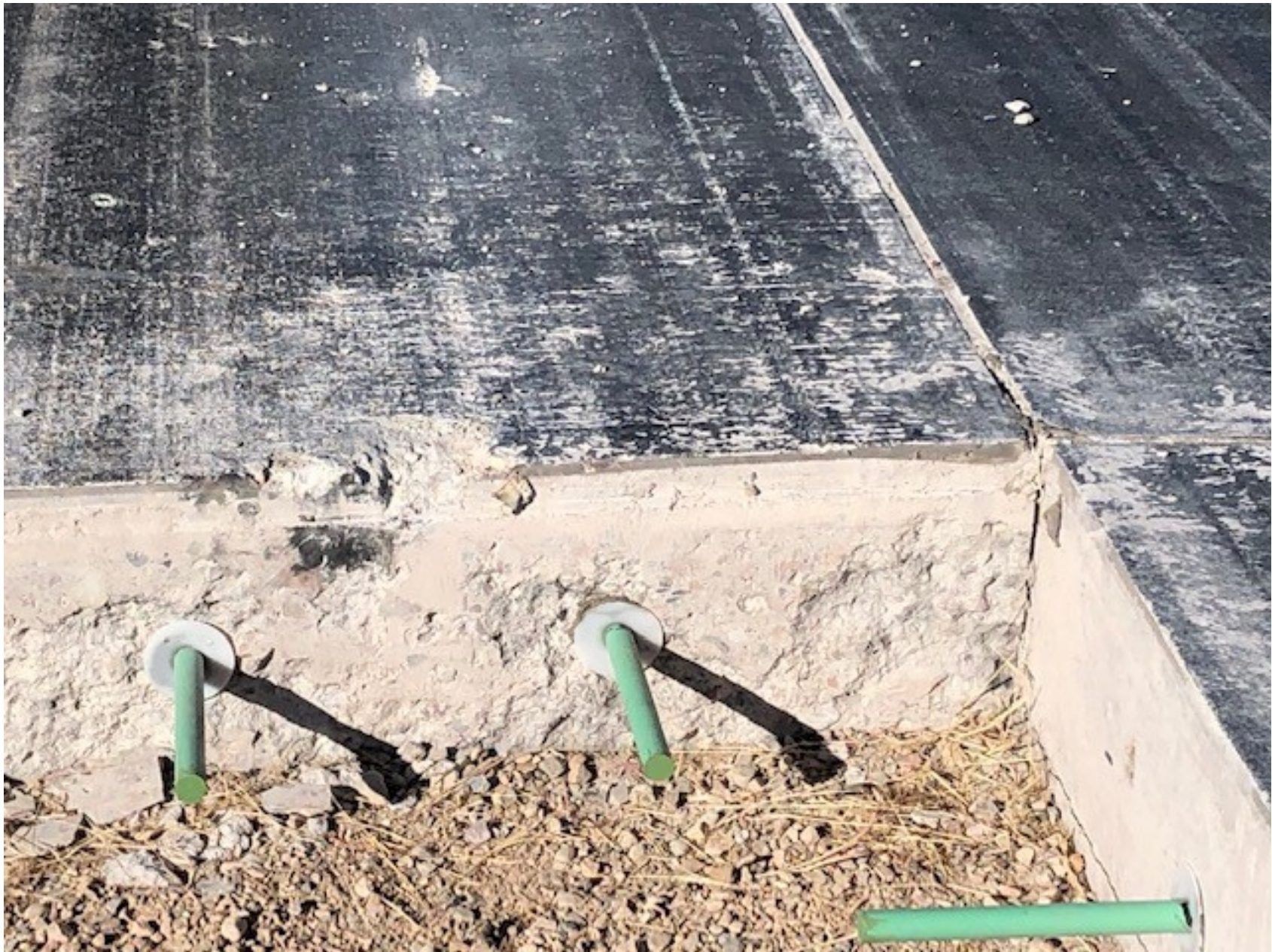
Photo 1 – View of runway trench which the left wheel struck during an attempted go around (courtesy of the operator)
